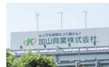
Wind power generation system
