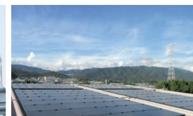
Solar power generation system
