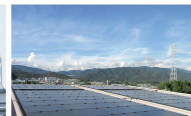
Solar power generation system
